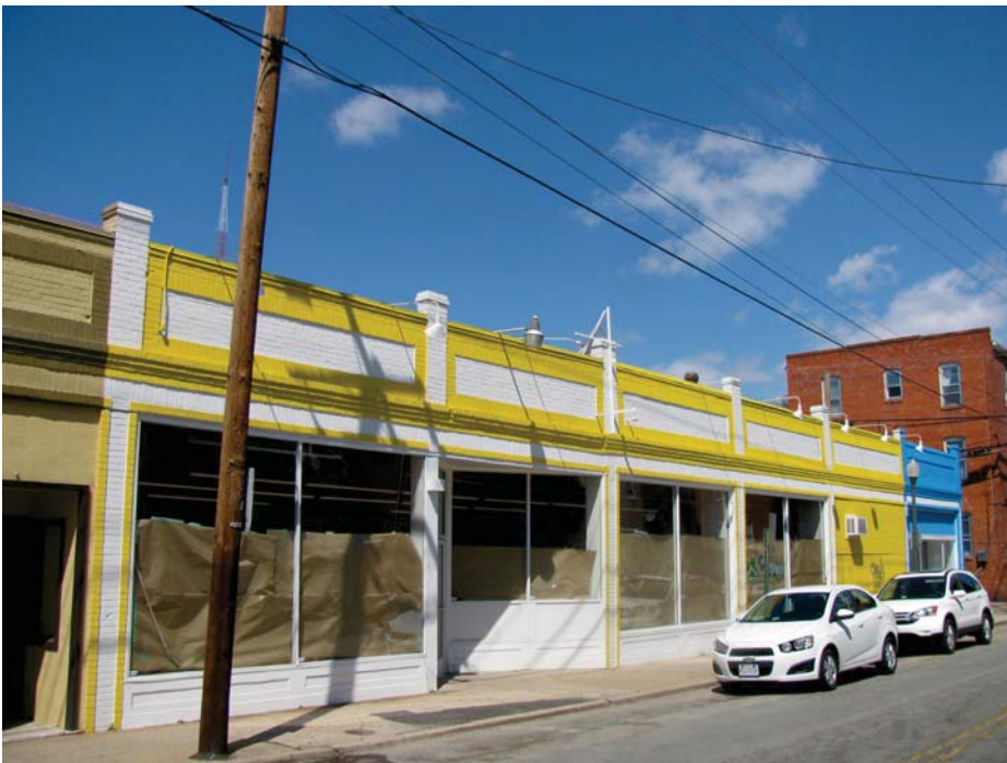
Image 25: 704 N. Sheppard Street has been vacant since November, 2013, but has historically been occupied by a neighborhood grocery market.
